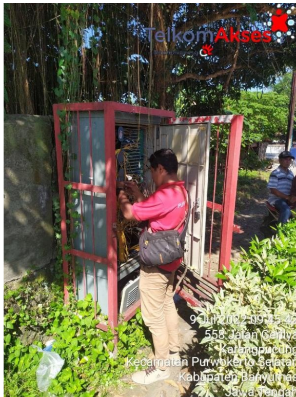
Gambar 2.2 ODC ( Optical Distribution Cabinet )
