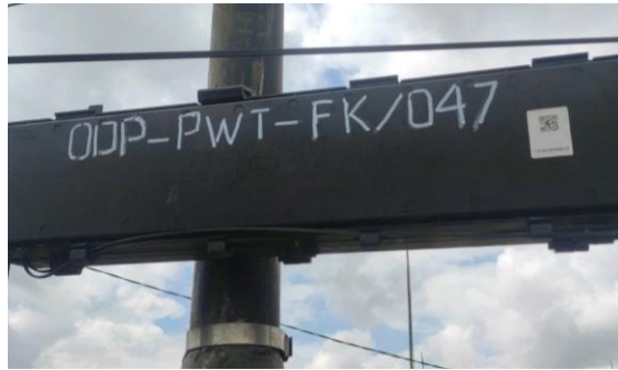
Gambar 2.3 ODP ( Optical Distribution Point )
