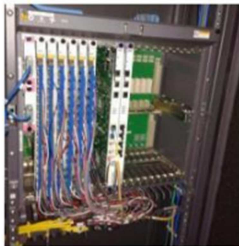
Gambar 2.1 OLT ( Optical Line Terminal )
