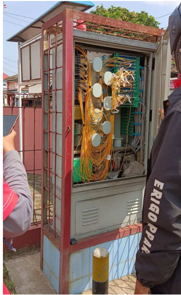
Gambar 2.3 ODC ( Optical Distribution Cabinet )
