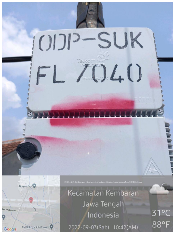
Gambar 2. 8 Optical Distribution Point Pole
