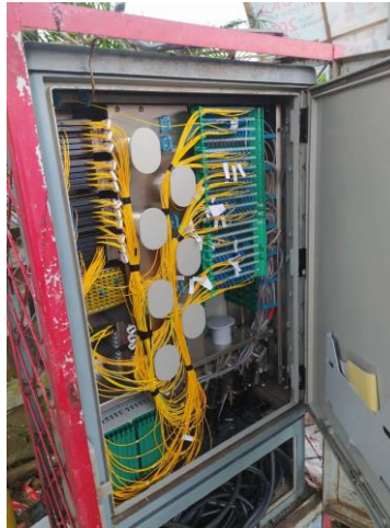
Gambar 2. 4 Optical Distribution Cabinet (ODC) [6]
