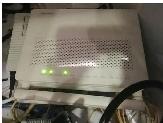
Gambar 2.2.11 Optical Network Termination [4].
