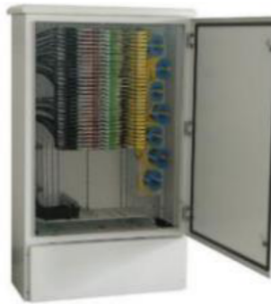
Gambar 2.2.3 Optical Distribution Cabinet
