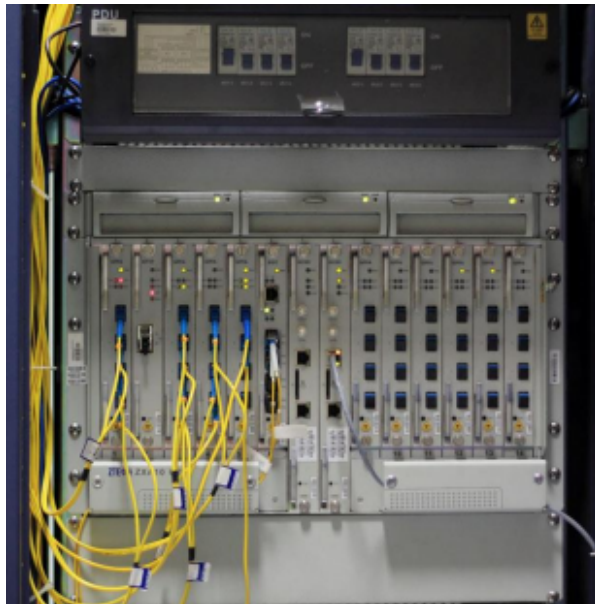
Gambar 2.3 OLT ( Optical Line Terminal )
