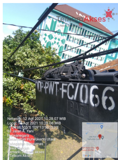
Gambar 2.5 ODP ( Optical Distribution Point )
