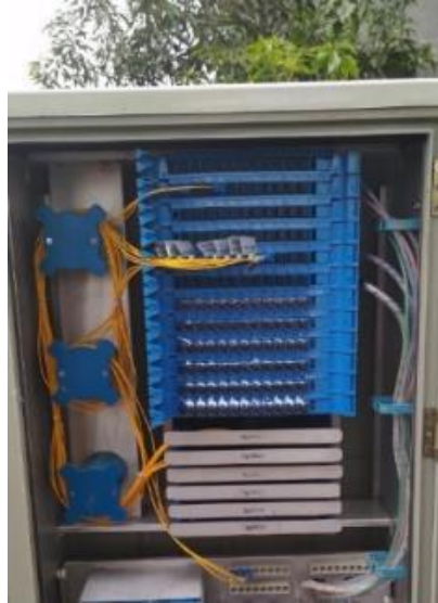
Gambar 2.3. Optical Distribution Cabinet
