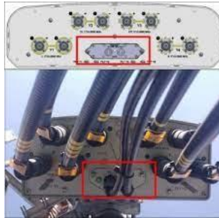
Gambar 2.6 Electrical Tilting Antena [3].
