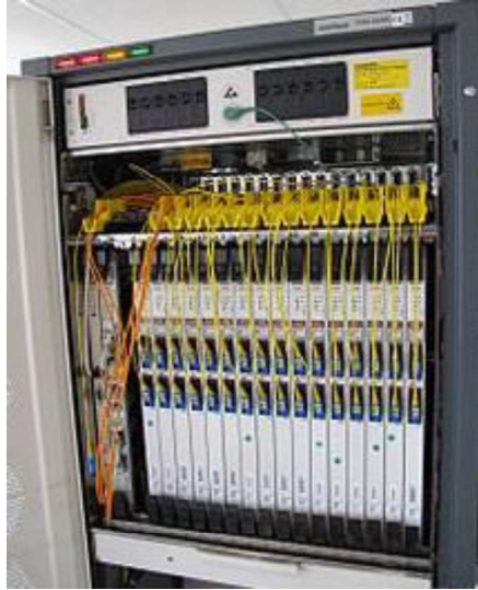
Gambar 2. 10 Optical Line Termination (OLT) [10]
