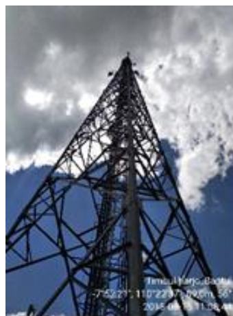
Gambar 2.4 Base Transceiver Station (BTS)
