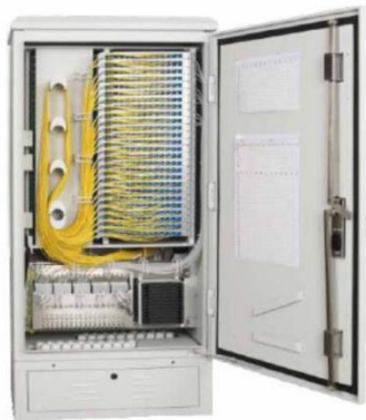
Gambar 1.12 Optical Distribution Cabinet [11]
