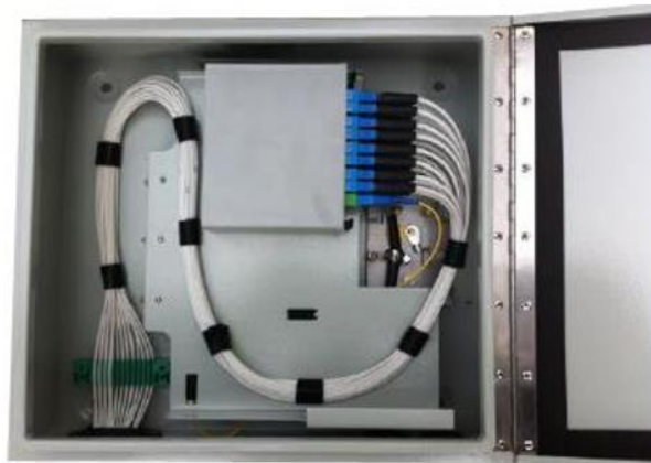
Gambar 2.13 Optical Distribution Point (ODP) [4]
