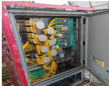
Gambar 2.3 Optical Distribution Cabinet [3].
