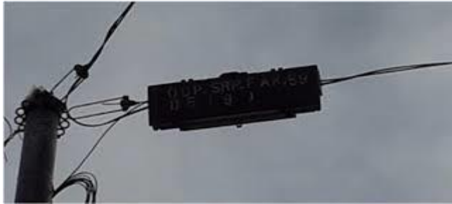
Gambar 2.2 Optical Distribution Point [3].
