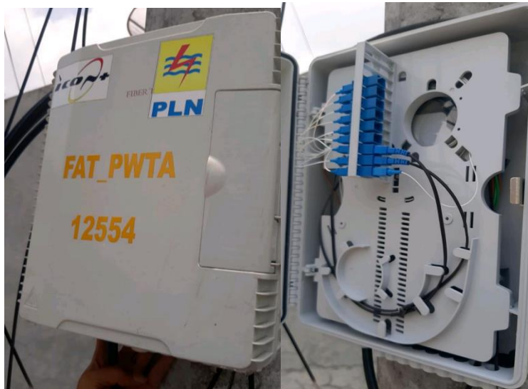
Gambar 2.4 Optical Distribution Point
