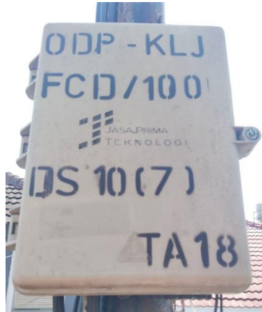
Gambar 2.10 ODP ( Optical Distribution Point )
